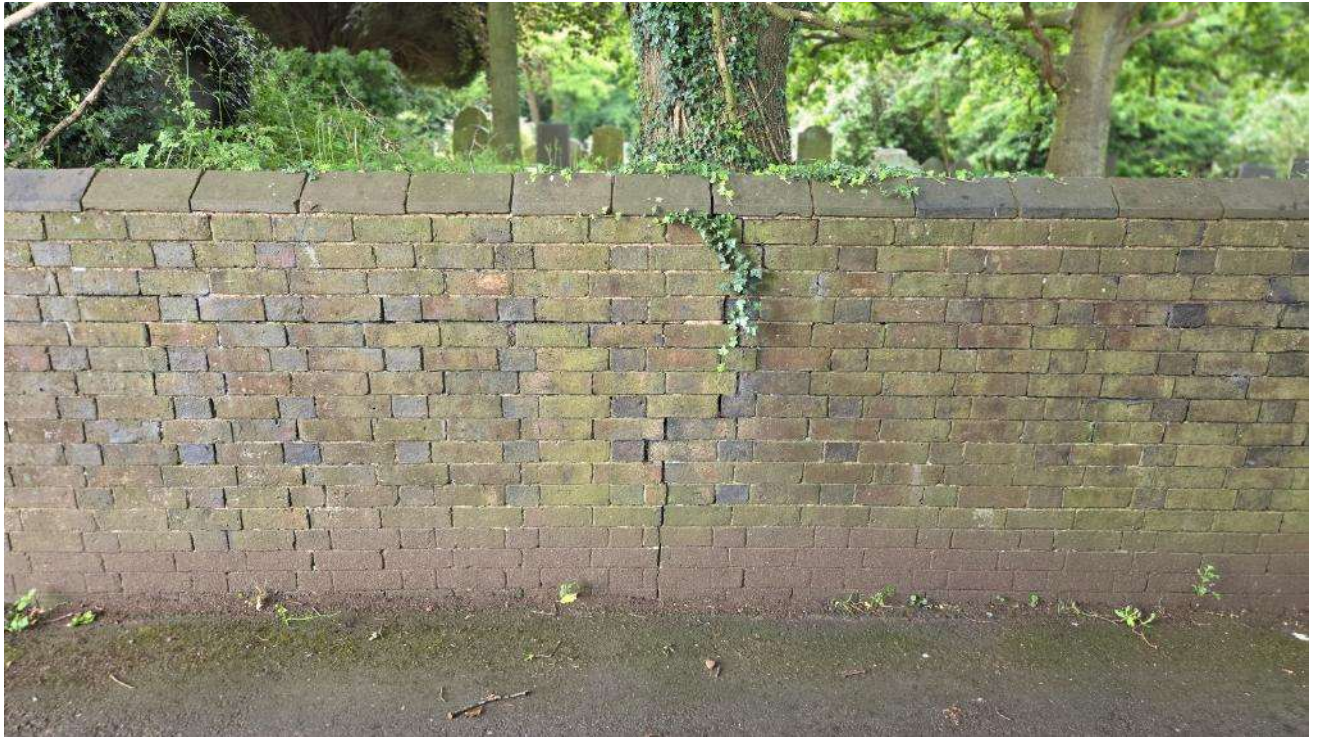
32) Near vertical crack further to the east in front of tree.
