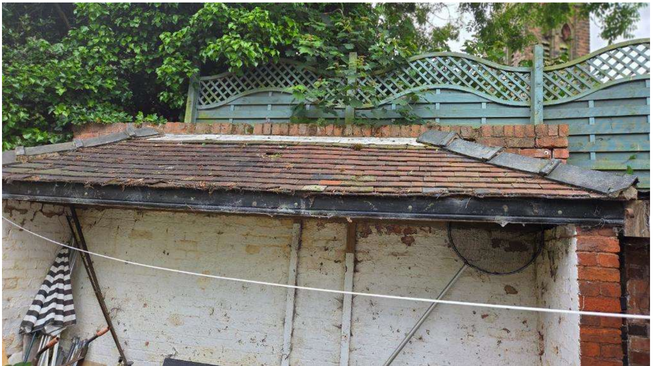
11) Open sided “store” with cracks to top of the wall by the fence.
