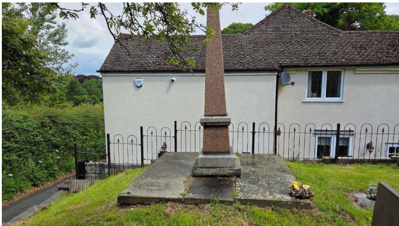
2) View looking north with base of grave settling and displacing slightly.
