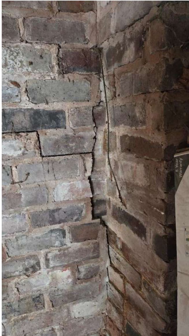
8) Cracking and displacement of wall adjacent to return brickwork at west end of outbuilding
