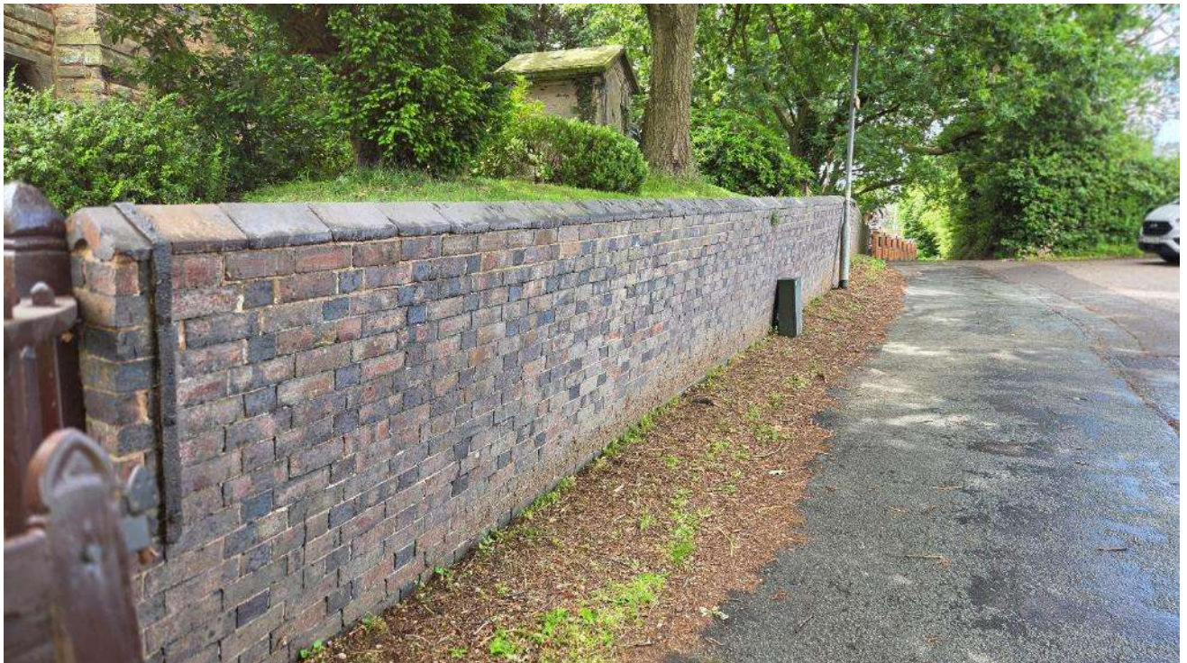
29) Retaining wall leaning towards lamppost leans further.
