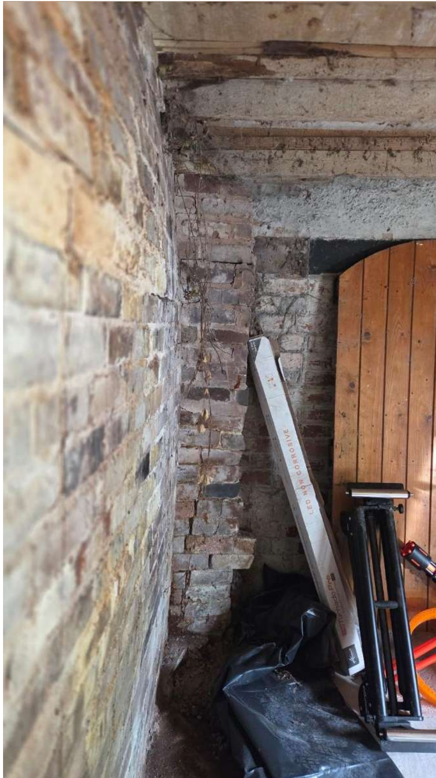
7) Bulge in retaining wall looking west, with cracked buttress wall to Cottage.
