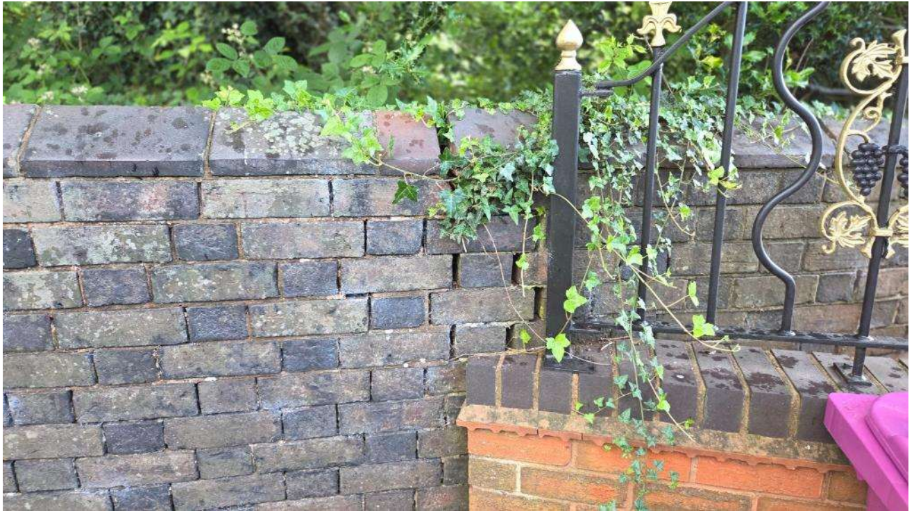
36) Open joints and slight movement where Green Fields wall is partly built into retaining wall.
