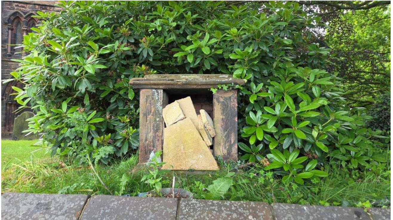
38) Cracked stonework to “tomb” facing Church Lane
