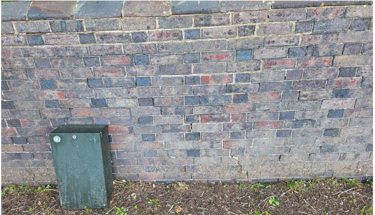
30) Leaning wall section with diagonal and vertical cracking from base as section to right and lamppost
