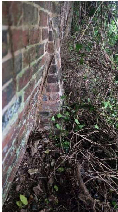
18) Small buttress with wall at base having rotated towards garden.
