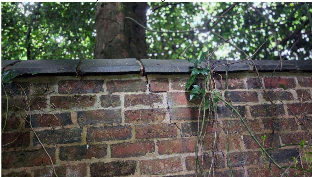
17) Minor crack through mortar joints and coping stone joints.
