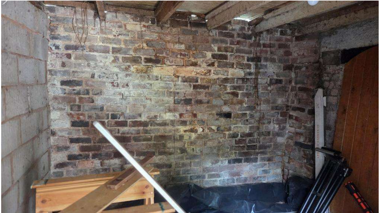
5) Rear wall of outbuilding forms the boundary retaining wall. Wall is bowed and cracked.
