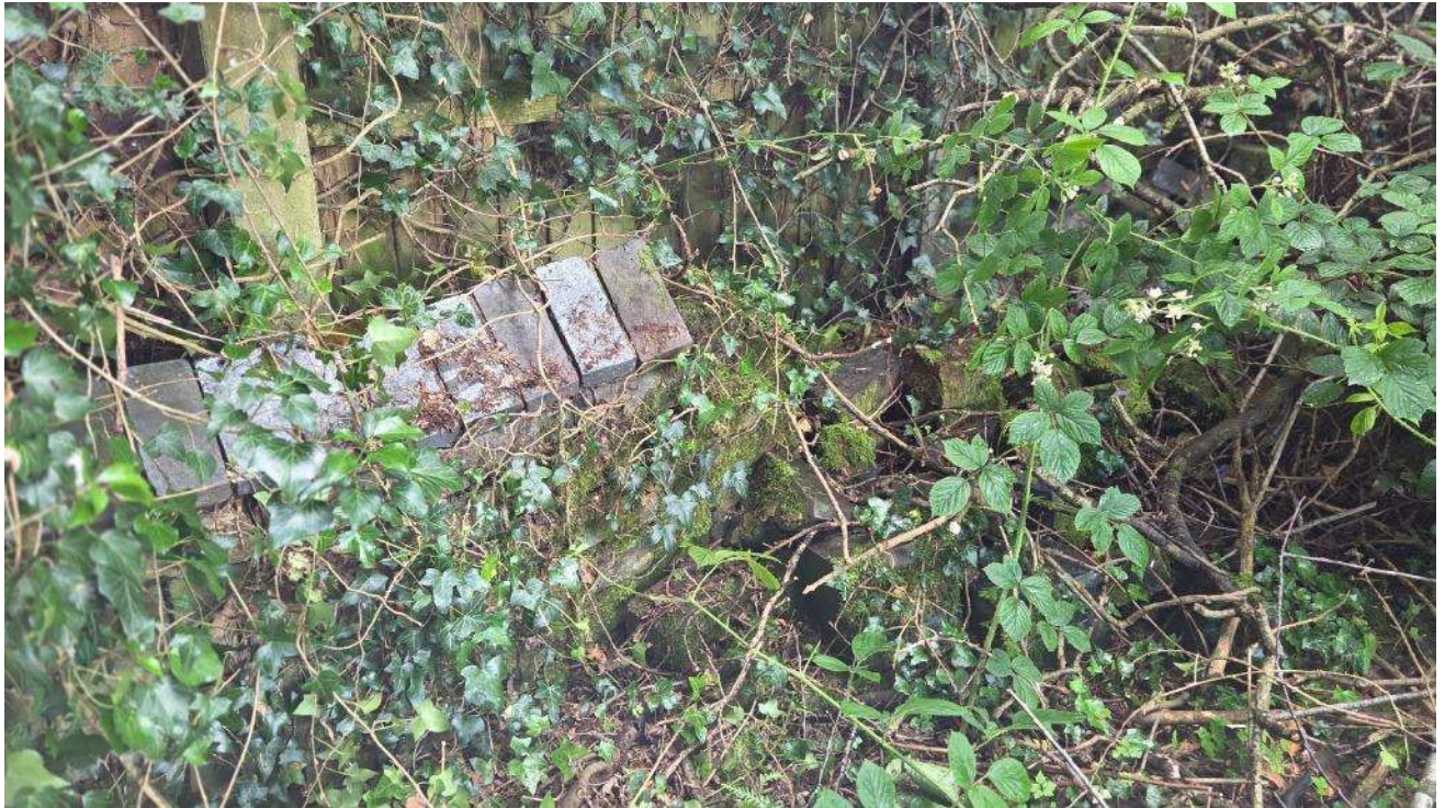
46) Collapsed top section boundary wall to the south retaining some ground with fence line of adjacent Green Fields close to the rear of the wall.
