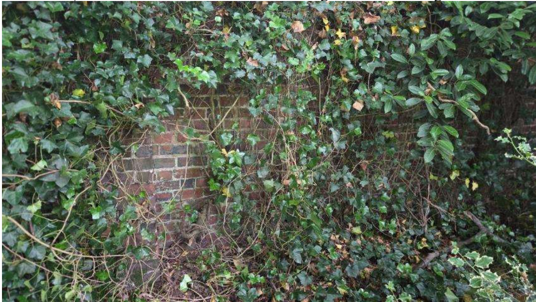
19) Typical vegetation growth from both churchyard side and garden with minor cracks and loos of mortar at cleared patch.
