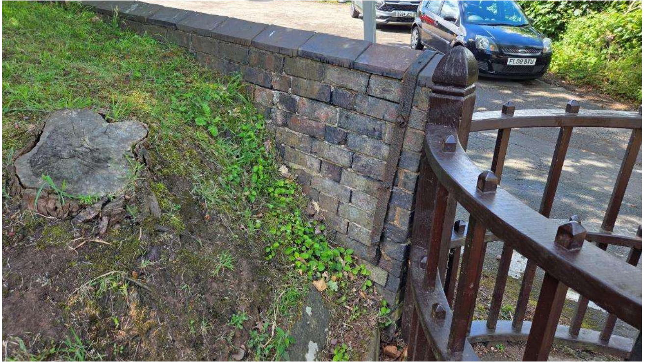
28) Entrance gateway with wall pushed by previous tree growth. Older iron strap bolted to end of the wall. Wall rapidly retains ground.
