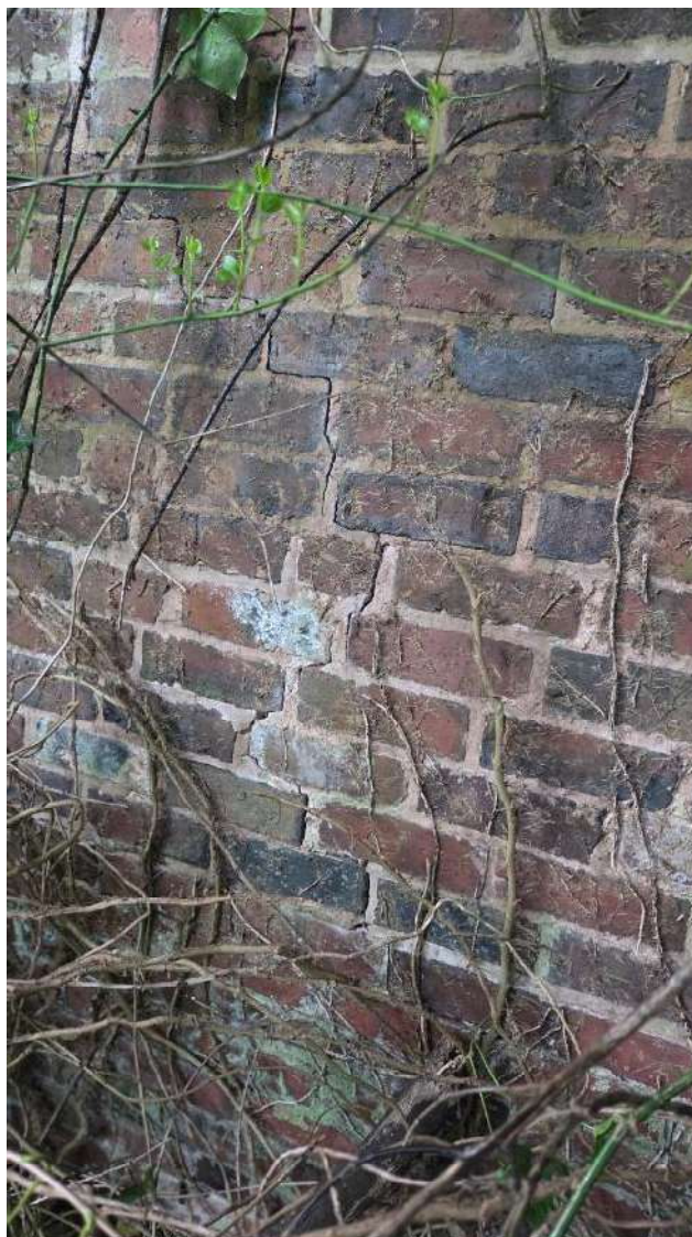
16) Further cracks along wall to the east.
