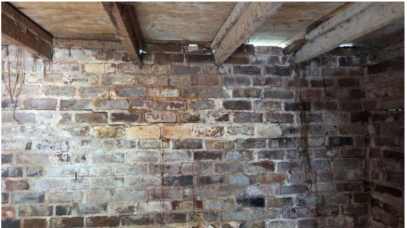
6) Horizontal cracks to face of retaining wall.
