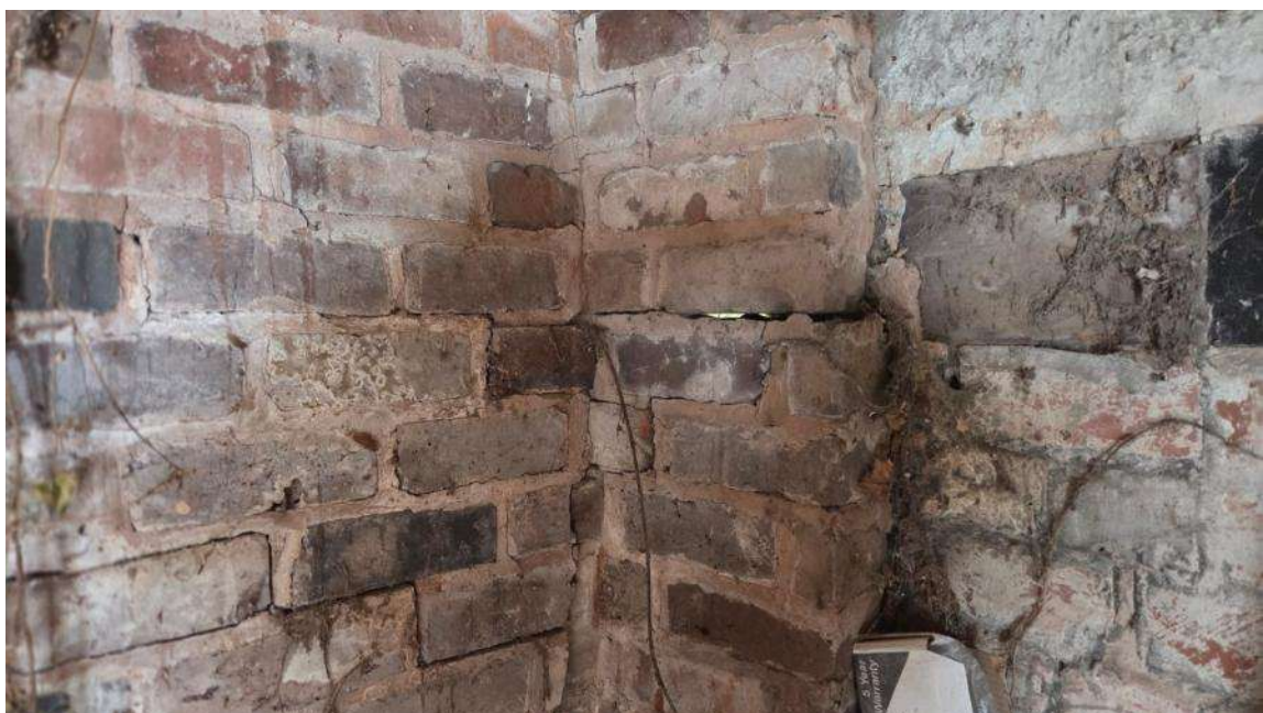
9) Further view of cracking and wall displacement at the west corner.
