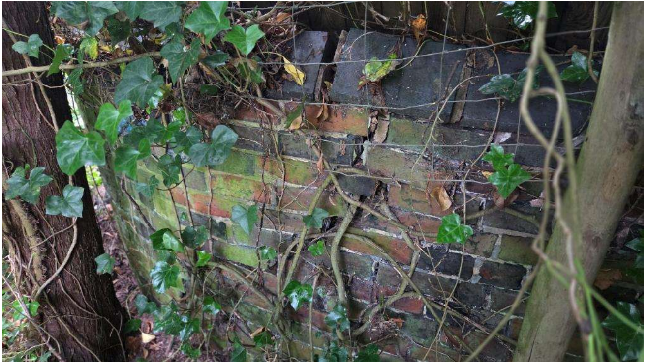
20) Severely cracked and rotated lower wall section at the NE corner.
