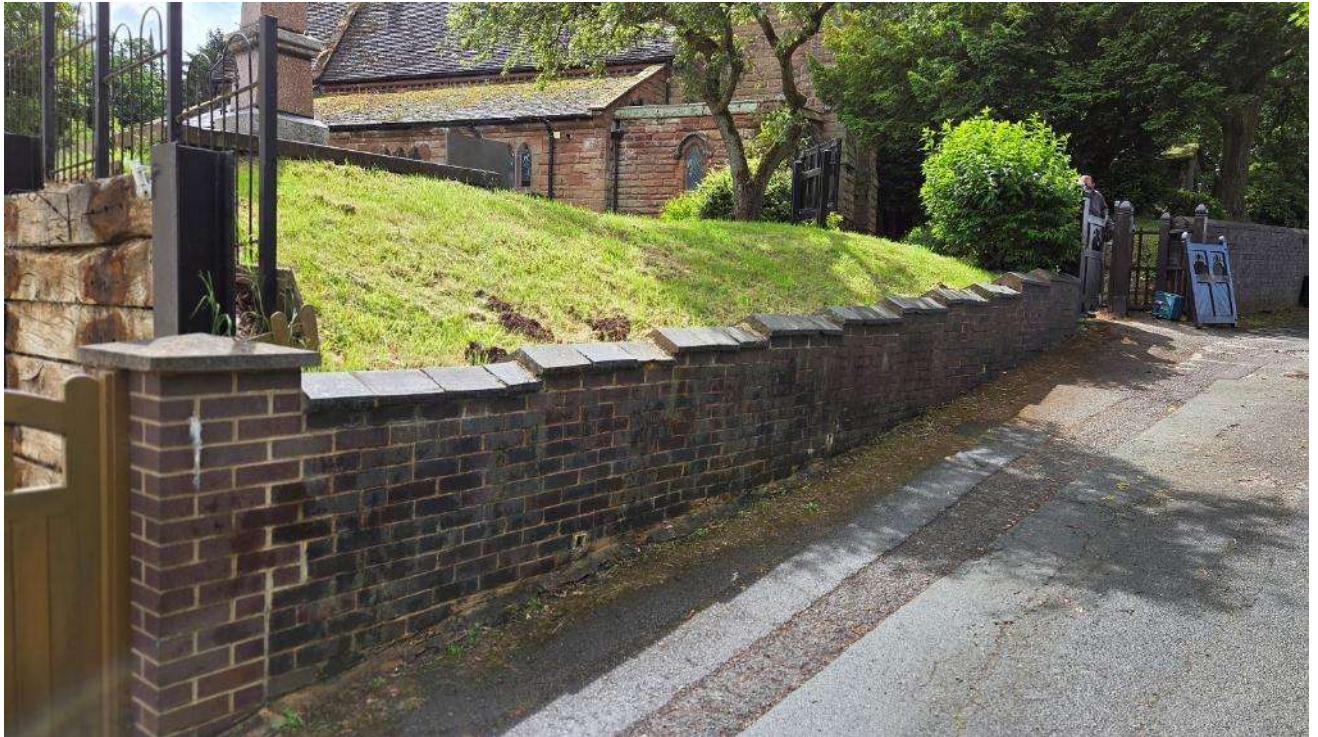
26) Church Lane elevation northern section stepped brickwork with newer looking weepholes.
